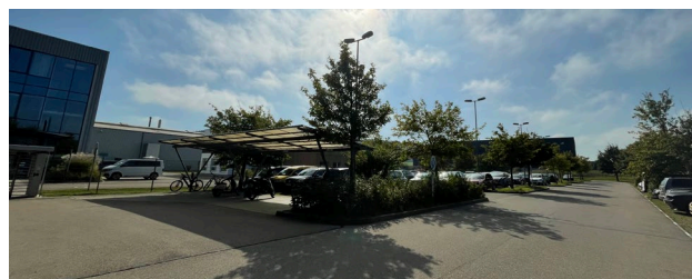
Figure 6: LED lighting in parking area in Neuburg, Germany
