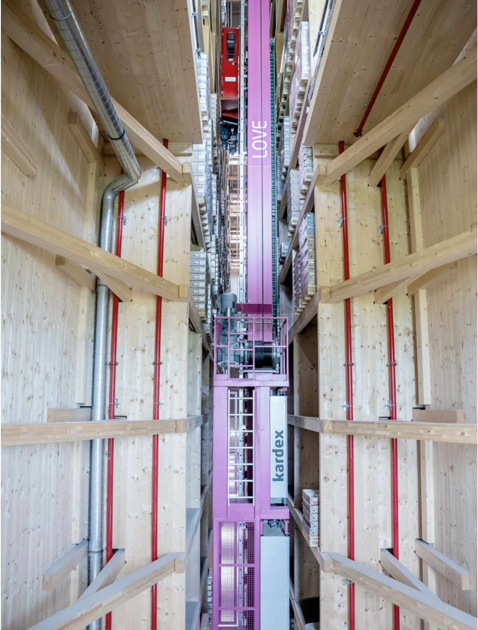
Weleda in Schwäbisch Gmünd, Germany, wooden rack combined with stacker crane by Kardex Mlog
